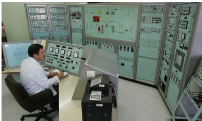
● Sala de Control del Reactor Nuclear Experimental Chileno 1, RECH-1
